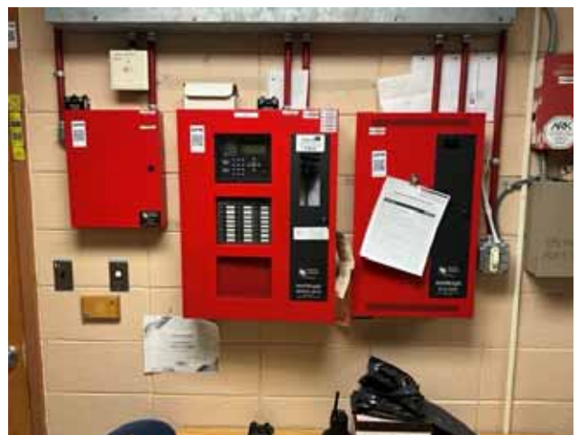
24 - FIRE ALARM PANEL
