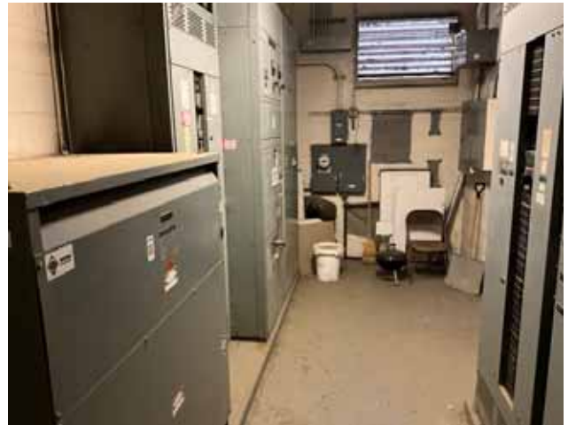
22 - MAIN ELECTRICAL ROOM
