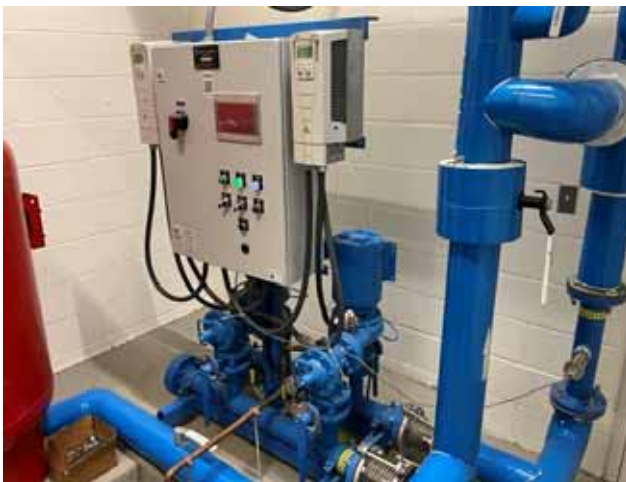
17 - DOMESTIC WATER PIPING
