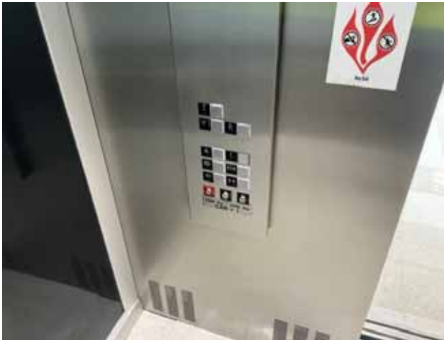
15 - ELEVATOR CAB PANEL
