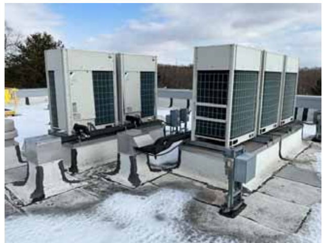
18 - ROOFTOP MECHANICAL EQUIPMENT
