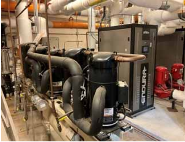
19 - MAIN MECHANICAL ROOM
